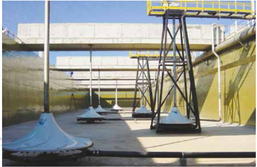
8 out of 22 HYPERCLASSIC® -Mixer/Aerators in a large municipal wwtp in São Paulo, Brazil
