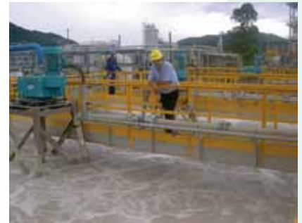
5 HYPERCLASSIC® -Mixing & Aeration Systems in an industrial wwtP in Brazil (Chemical Industry)
