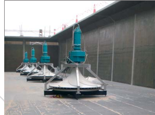
HYPERDIVE® Mixing & Aeration System during installation in a municipal wwtP in Middle East
