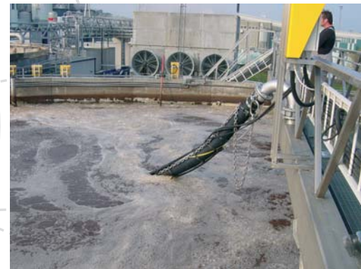
HYPERDIVE® Mixing & Aeration System in operation in an industrial wwtP in Sweden (Pulp & Paper Industry)
