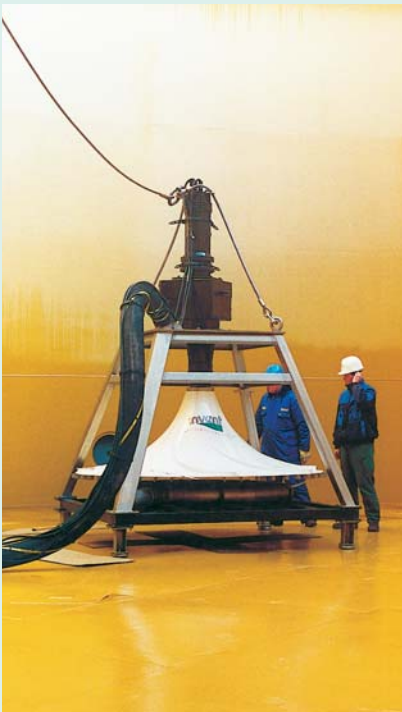
1 out of 4 HYPERDIVE® Mixing & Aeration Systems at an industrial wwtp in the Netherlands (Oil & Gas Industry)
