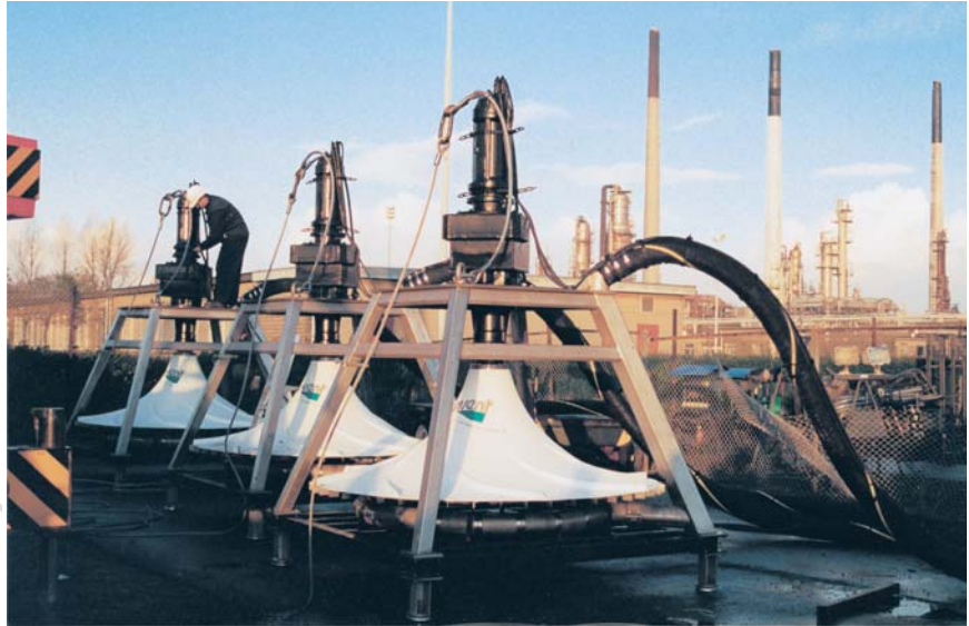
3 out of 4 HYPERDIVE® Mixing & Aeration Systems at an industrial wwtp in the Netherlands (Oil & Gas Industry)
