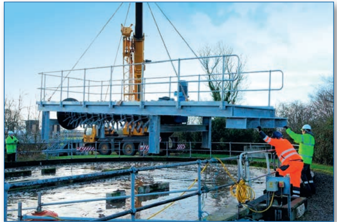
Commissioning at site
