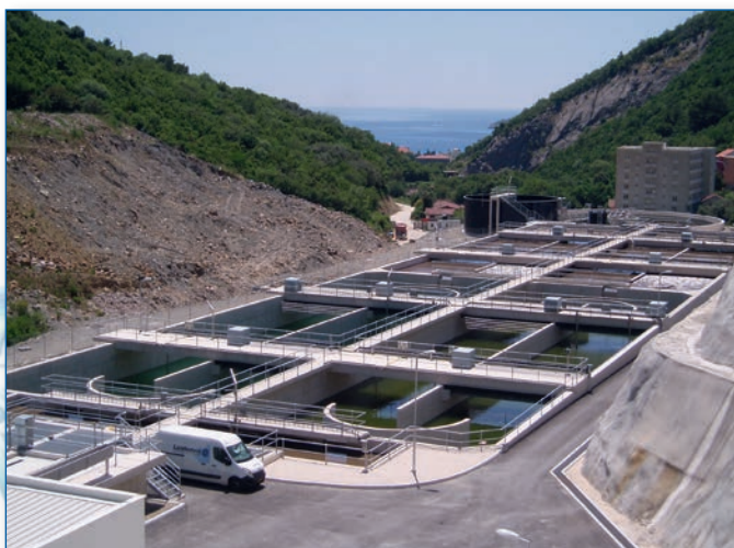
Landy brush aerator at WWTP Budva (Montenegro)
