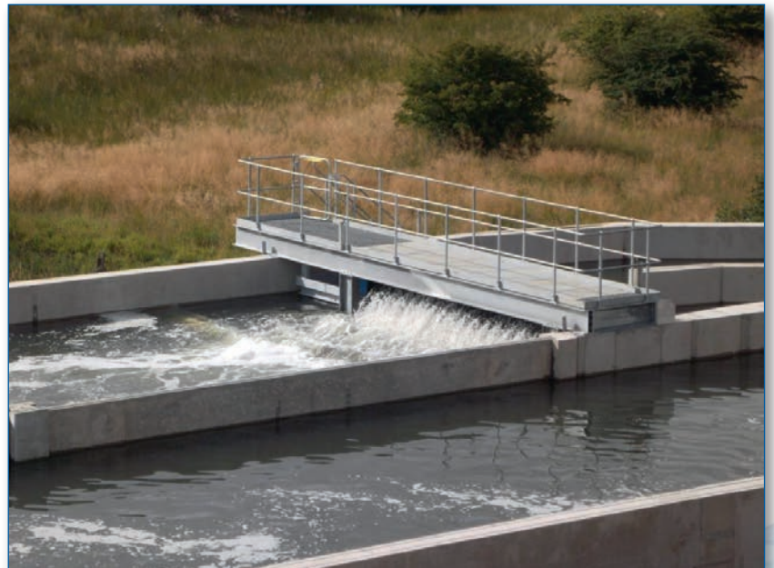
Landy brush aerator mounted underneath steel bridge
