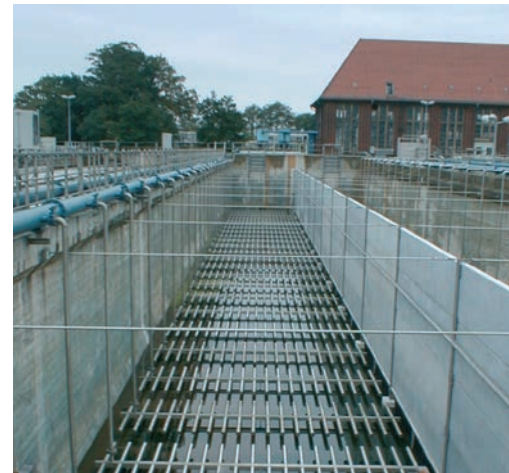
TEX-FLEX aeration system in a municipal wastewater treatment plant in Germany
