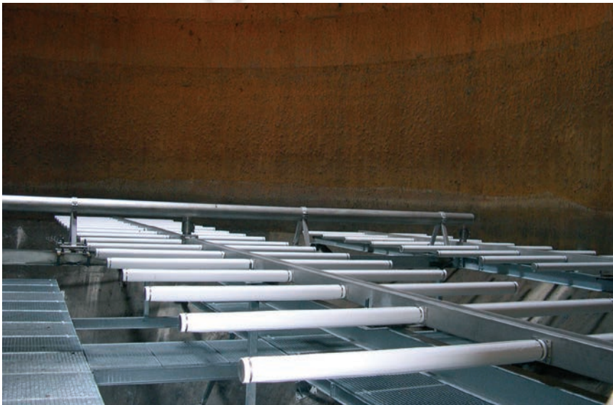
TEX-FLEX aeration system in a municipal wastewater treatment plant in Belgium
