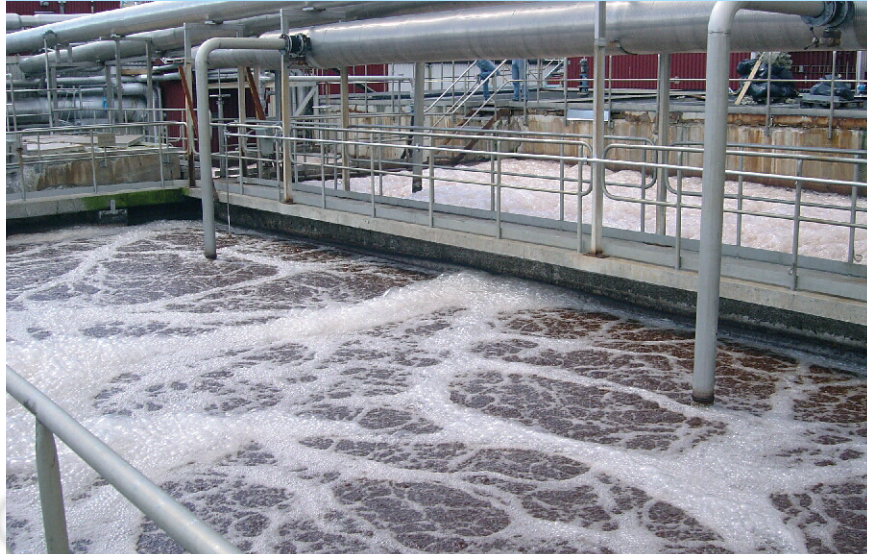
TEX-FLEX aeration system in an industrial wastewater treatment plant in Sweden (Pulp & Paper Industry)
