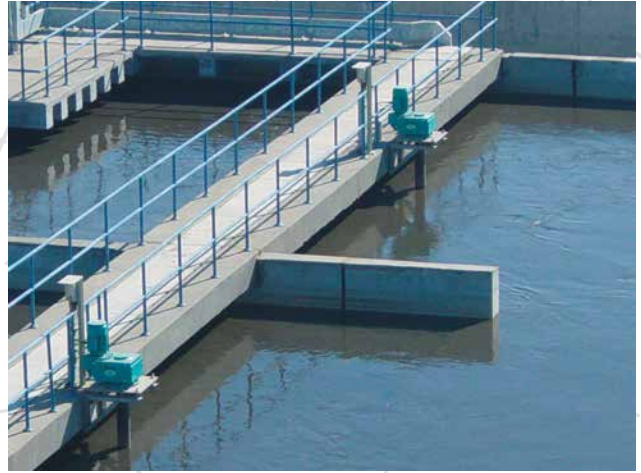
2 out of 45 HYPERCLASSIC® -Mixers in a wwtp in Kuwait City, Kuwait
