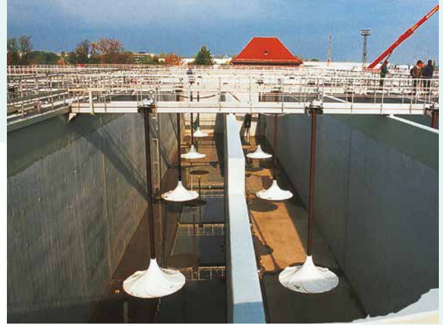
7 out of 33 HYPERCLASSIC®-Mixers in a wwtp in Berlin-Stabnsdorf, Germany
