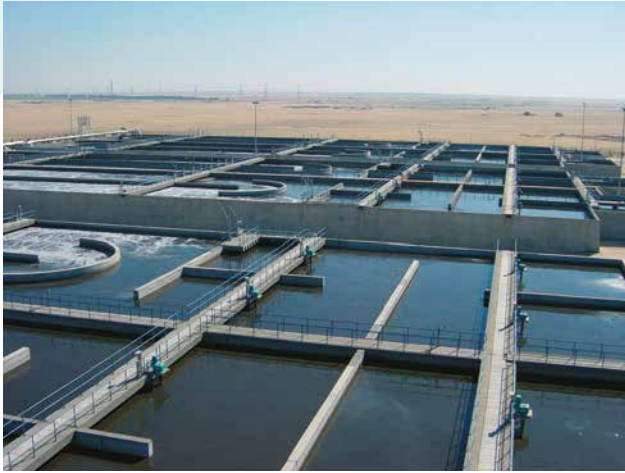
45 HYPERCLASSIC® -Mixers in a large wwtp in Kuwait City, Kuwait
