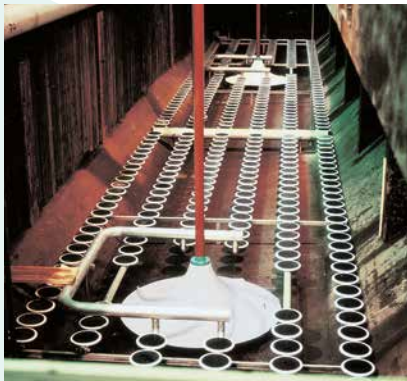
2 out of 48 HYPERCLASSIC® -Mixers in a wwtp in Stockholm, Sweden
