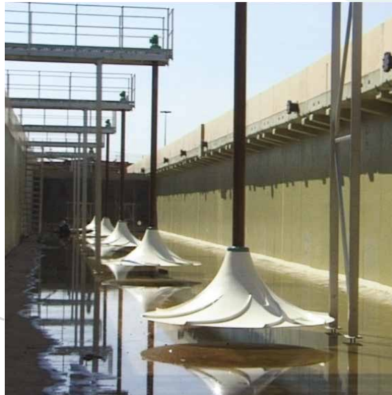
6 out of 120 HYPERCLASSIC® -Mixers in a wwtp in Berlin, Germany
