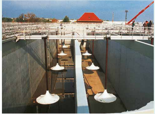
7 out of 33 HYPERCLASSIC®-Mixers in the wwtp Berlin-Stabnsdorf, Germany
