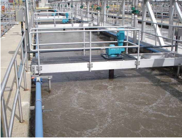
3 out of 90 HYPERCLASSIC®-Mixers in the wwtp Bowery Bay, New York, USA
