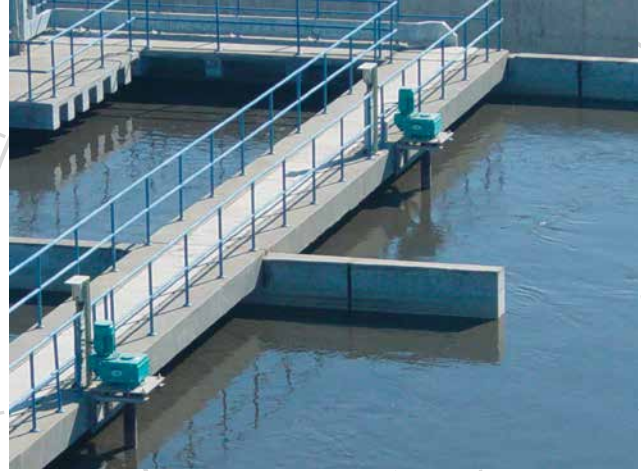
45 HYPERCLASSIC®-Mixers in the wwtp Sulaibiya, Kuwait-City, Kuwait
