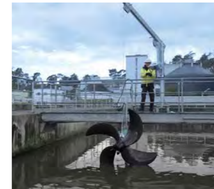
Maintaining a CYBERFLOW ® -Accelerator in a municipal wwtp in Germany
