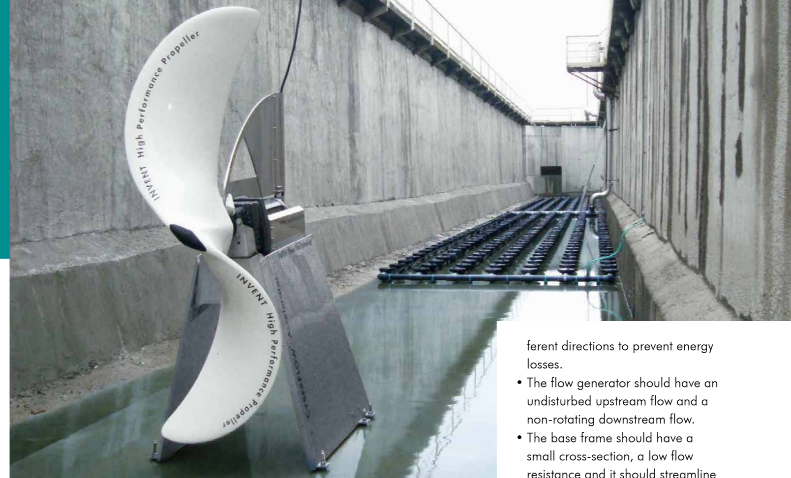
CYBERFLOW®-Accelerator in a municipal wwtp in Bulgaria
