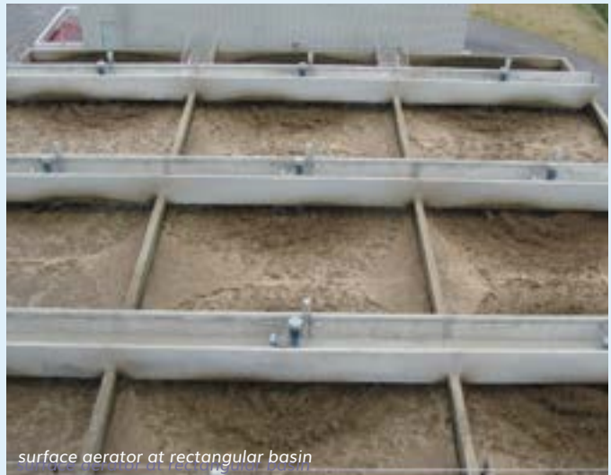
floating surface aerator
